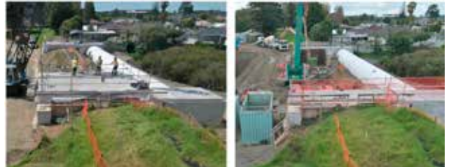
Left: Old pipe inside embankment. Right: Old pipe has been removed and sewage is now flowing through a temporary diversion pipe.
