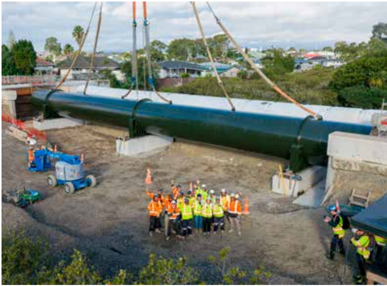
NZ's largest pipe lift this year, at Harania Creek. Photo by @cuetonemedia / Cuetone Media.
